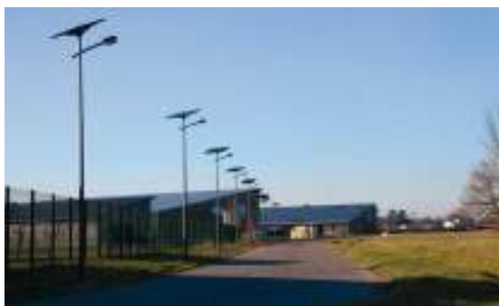
Eclairage public de route en LED
