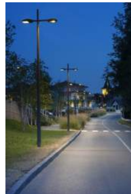
Eclairage public de route en LED
